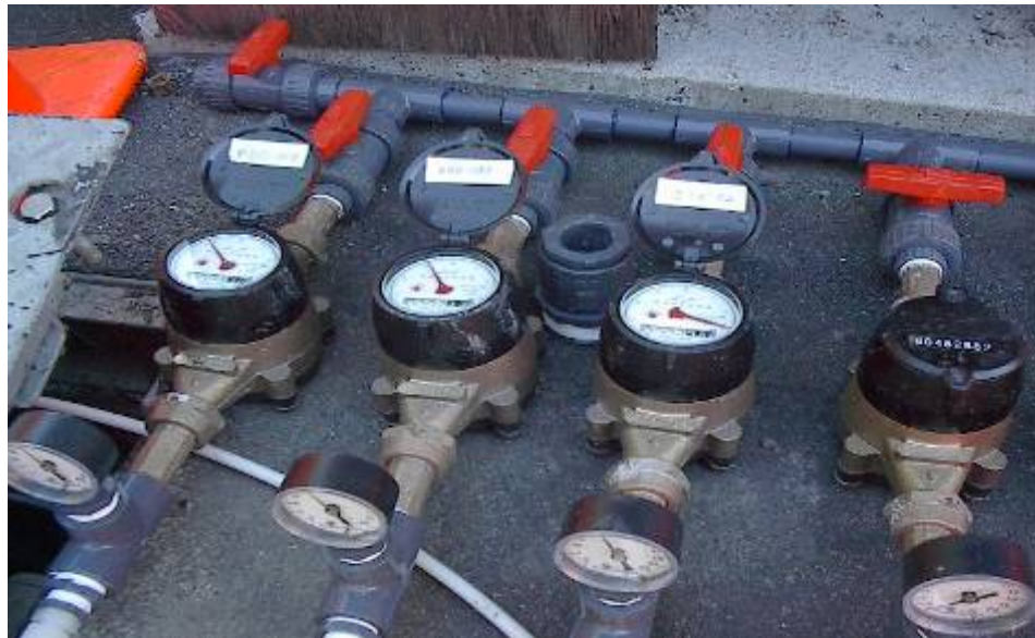
Figure 5.10 Injection System Manifold Showing Separate Control Valve and Flow Totalizer for Each Injection Well (Photo courtesy of EOS Remediation, Inc.)
