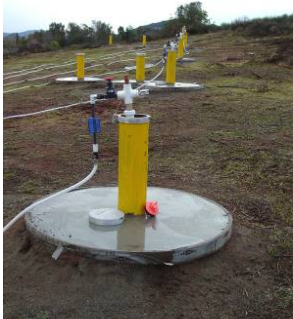
Figure 5.9 Typical Well Head Configuration (Photo courtesy of Remediation and Natural Attenuation Services, Inc.)
