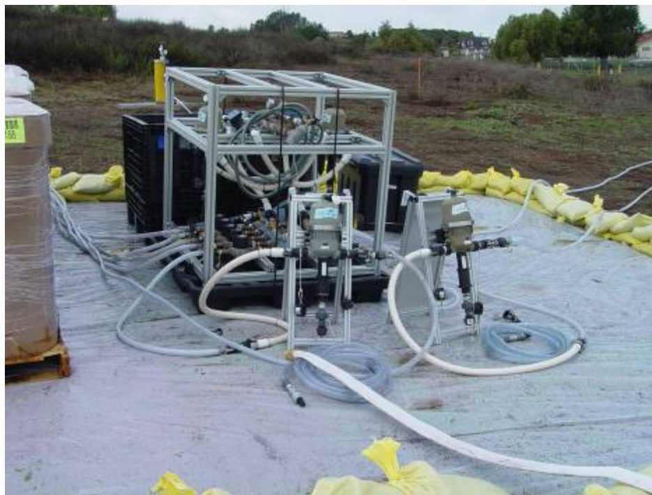
Figure 5.11 Proportional Feed System for a 10-Line Injection System (Photo courtesy of Remediation and Natural Attenuation Services, Inc.)
